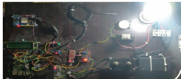
Fig. 12. Transformer Without Fault
