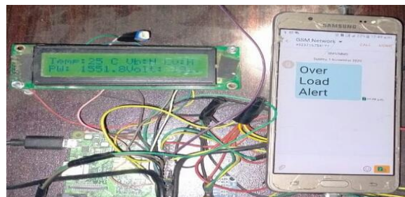
Fig. 6. Fault Due to overload
